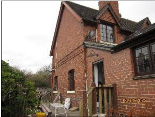
Photograph again showing the existing north elevation of the dwelling, which is where the proposed side extension will be located.
